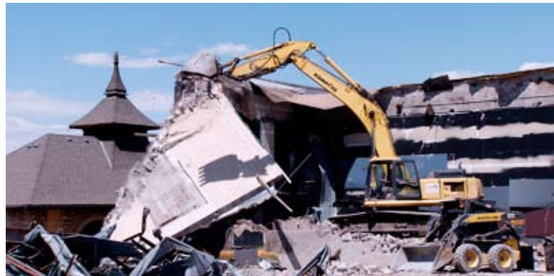
Figure 1: This slow-motion shot of the wall of a building being torn down – ACG-FH101-08 on Artbeats FootageHub – is available at a maximum size of 2048x1152 pixels. The smaller size is a tradeoff for the drama of seeing it in slo-mo. However, there are still enough pixels to fit inside a 1920x1080 frame, with more than enough to pan and scale it inside a 720p, DI, or DV project.
